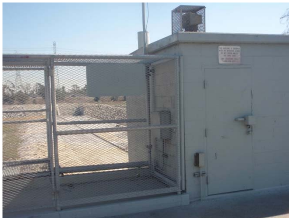
1. Unit connected to outfall from bike path
